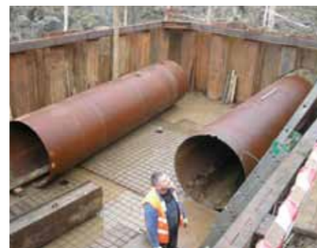
The first steel pipe DN 1,400 mm jacking before completion, jacked under the Czech Railway and the road towards the supply facility near the Ohře River.
